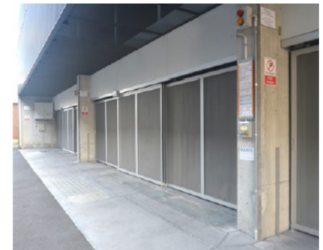
Figure 84. Self-actuating vertical-rise flood barriers South Melbourne laneway.
